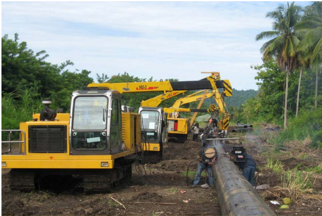
Position and welding of Slurry Pipeline – 75km of 135km completed Ramu Nickel-Cobalt Mine
