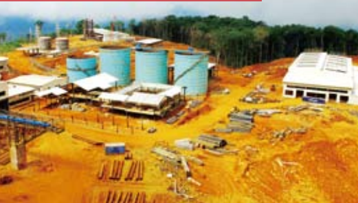
KBK mine site beneficiation plant
